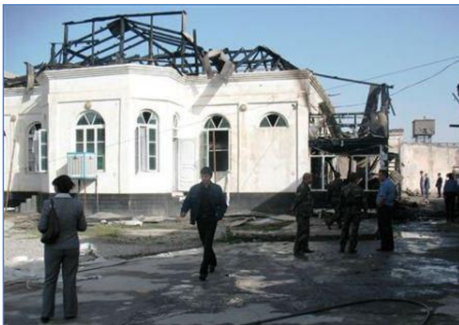
THE BUILDING, ADJACENT TO ISLAMIC RENAISSANCE PARTY’S HEADQUARTERS AND ITS MAIN PRAYER HALL, WAS ALMOST COMPLETELY DESTROYED BY FIRE ON THE AFTERNOON OF 23 OCTOBER 2010 (PHOTO: RFERL)
